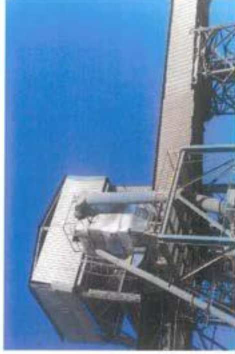
Installed Big Filters at Fly Ash Silo
