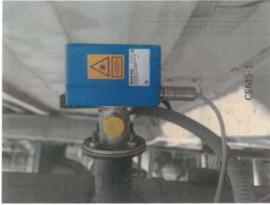
Annex.-4(Online CEMS in both Stacks)
